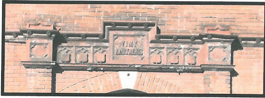
Before renovations to Vimy Apartments painted metal bas-relief plaque above front entrance approx. 12' lx3' h. Old green awning removed showing white keystone; keystones also top of third level windows. Photo May 2017.
