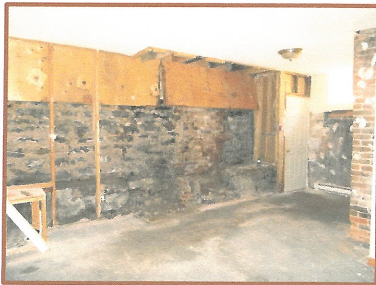
2015 November, Unit #1A before renovation along with vestiges of stone stairs that lead to old exterior staircase and since bricked over door to the one-time Annex and below showing after renovations. Photos 2015.
